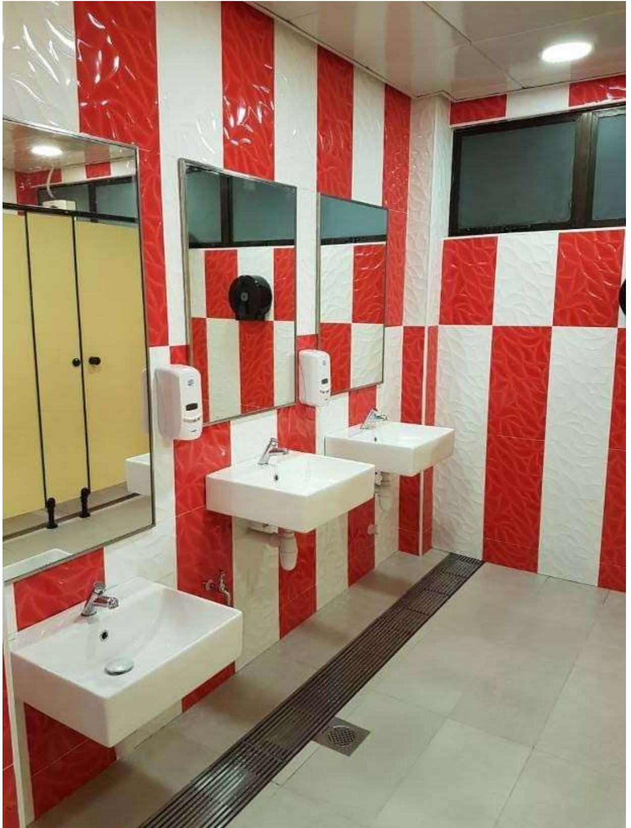
Illustration 15: Standalone wash basins (without vanity tops) and scupper drains with metal grating
